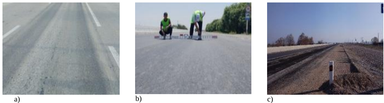
Fig. 1. Wheel-path rutting and pavement roughness deformations on the 1400–1420 km section of the M-39 “Almaty–Bishkek–Tashkent–Shahrisabz–Termez” highway
