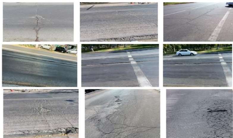
Fig-2. General View of the Major Pavement Distresses Identified on the Small Road in Tashkent City
